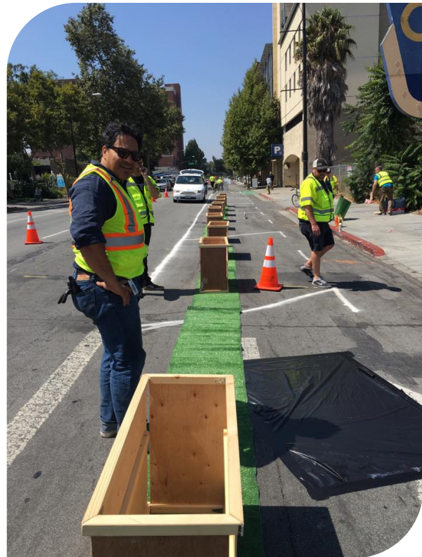
City of San Jose staff and volunteers install a temporary pop-up cycle track on Fourth Street to demonstrate the city's plans for a connected network of protected bikeways in downtown. The reusable, portable planter boxes were borrowed from Mountain View's local bicycle advocacy group, which loans them out for demonstrations like this one. Photo: Jessica Zenk
