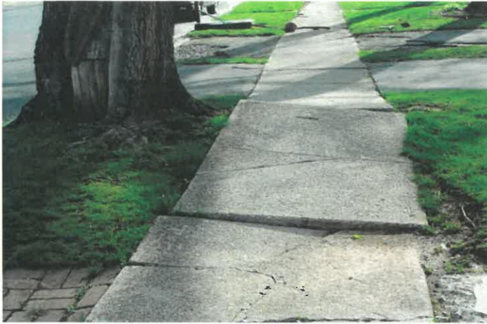
Broken sidewalk - Photo Credit: Medium
