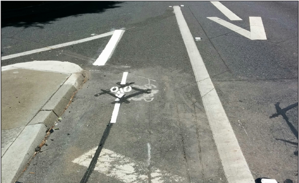
b. View of a bike detector embedded in a bike slot. The purpose of a bike detector is to detect a bicyclist approaching an intersection and communicate with the traffic signal cabinet to provide enough time for cyclists to safely cross an intersection.
