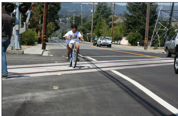
New concrete railroad crossing at Cox Avenue in Saratoga, funded by Measure B.
